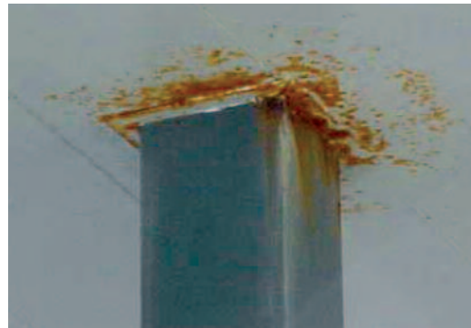
Treat rust and paint the canopy deck.
