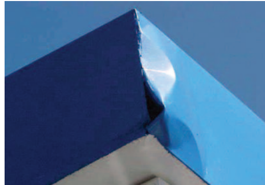
Repair damaged canopy elements.
