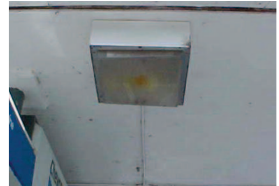
Repair and paint canopy and replace the dirty lens in under canopy light fixture.
