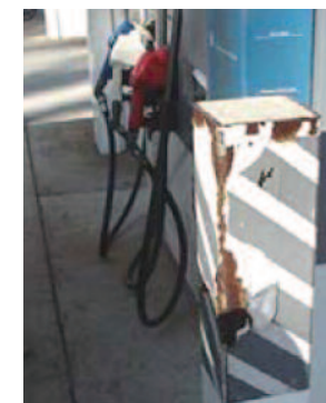
Paint and replace damaged/torn decals on worn bumper posts.
