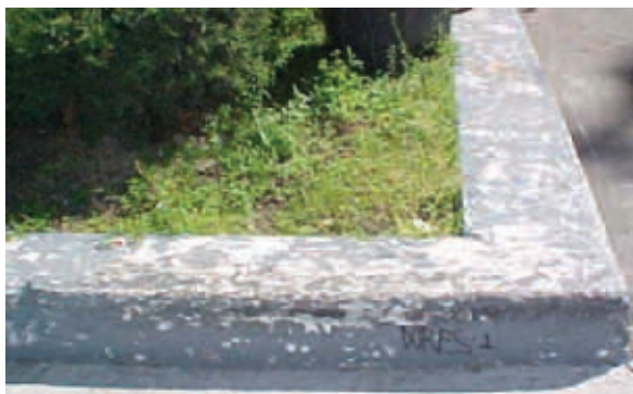
Paint faded and worn curbs.
