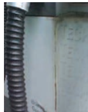
Treat rust and replace decal.
