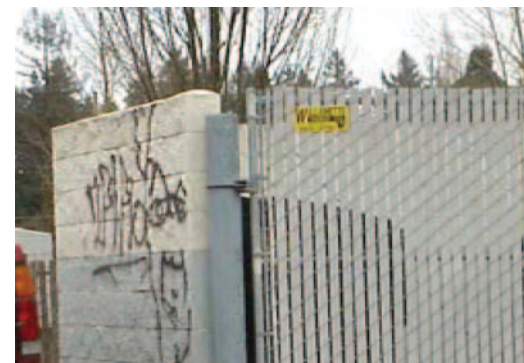
Remove or paint over graffiti.
