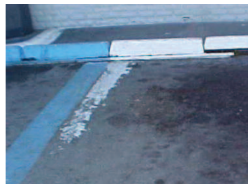
Repaint worn lot striping, and pressure-wash or treat oil and grease buildup.
