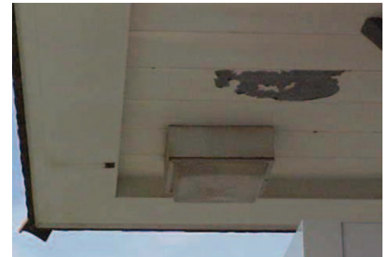
Repair and paint the canopy deck.
